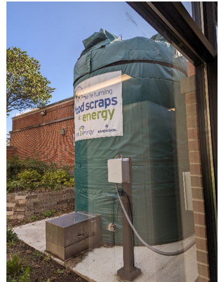
Figure 40. Holding tank for food scrap slurry outside of LAR Dining Hall.
